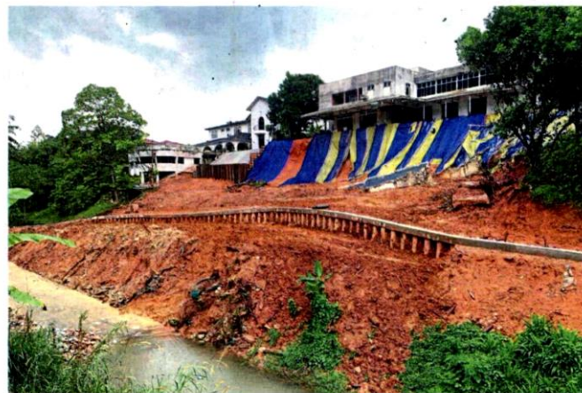
Some of the double-storey houses affected by the landslide along Jalan Kemensah Heights.
